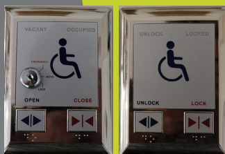
Disable Door Controller
