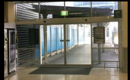
Sydney International Airport. Replace old with DSH 250 System.
